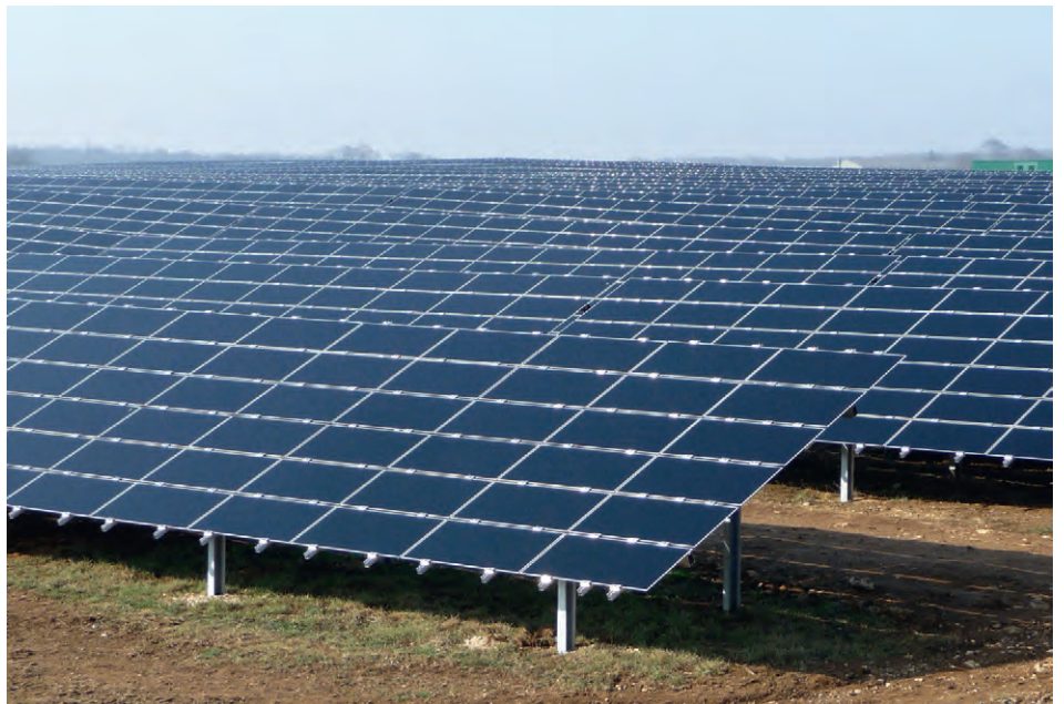
The Toul-Rosières photovoltaic power plants, located in Lorraine (France), co-financed by the 2020 European Fund for Energy, Climate Change and Infrastructure ("Marguerite") - crédits : Pierre Gerbeaud
